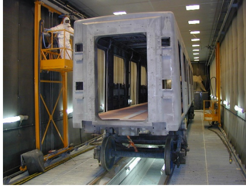
Figure 19 Blasting rooms (abrasive cleaning).
