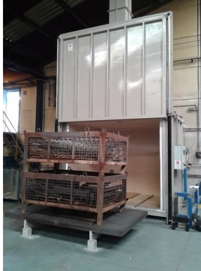
Figure 11 Industrial furnace (thermal cleaning).
